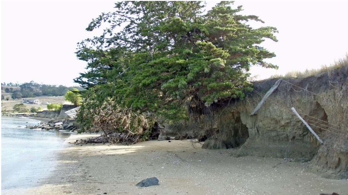
Figure 14: An eroding soft rock (cohesive clay) shoreline at Rokeby Beach (Storm Bay region). This is a soft rock shoreline for which historic recession rate data is available from aerial photography. Photo by C. Sharples.
